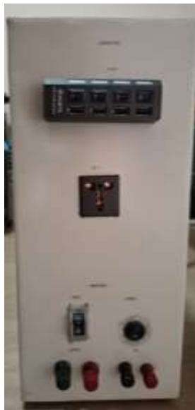
Gambar 4. Panel PLTS Tampak Samping
